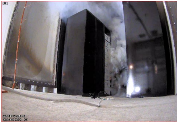
Smoke accumulation [TR + 00:00:31]
