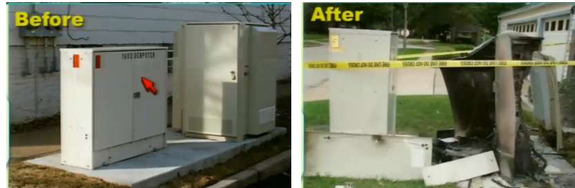
Telco cabinets w/ Li-ion backup (mid-2000s)
